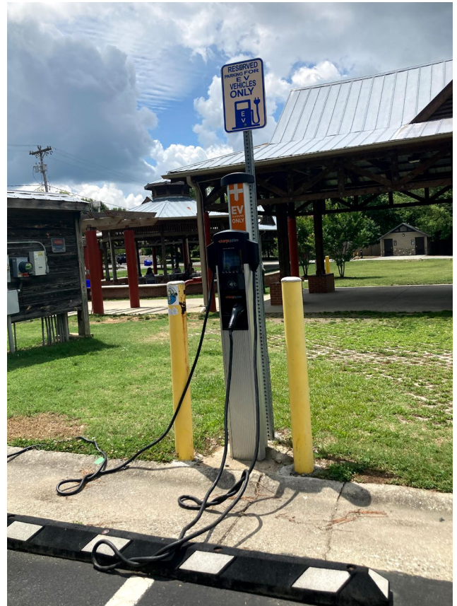
▲ Electric vehicle charging station at Town Commons
